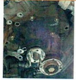
Old, leaking water pump
